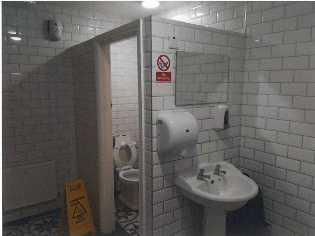
Images of new toilets, male and female relocated into the former lounge area.
